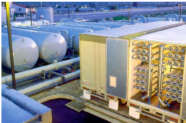
Figure 1: Seawater desalination facility, Santa Barbara
