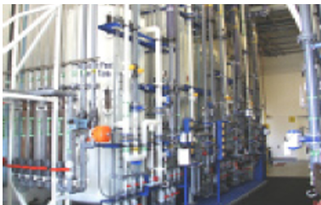
Figure 2: Interior of the plant
