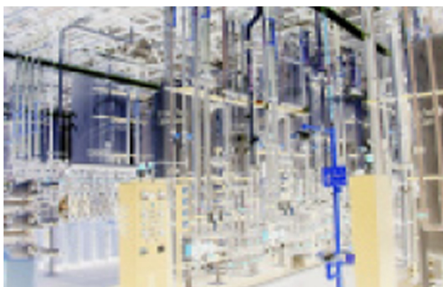
Figure 3: Interior of the plant
