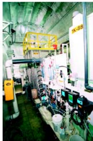
Process equipment skid with membrane tank in background.
