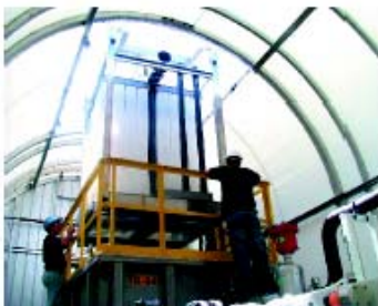
Hollow-fibre membrane cassette being lowered into tank. The surface area of the membrane is 758.4 m 2 .
