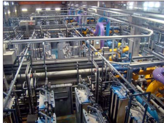
Figure 1: EDR water treatment plant at ATLL
