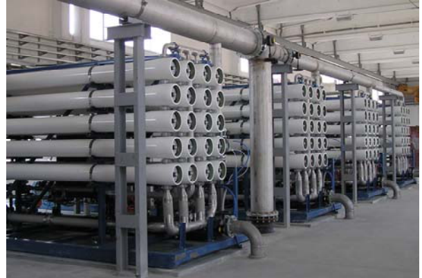
Figure 1: PRO Series RO units installed on site
