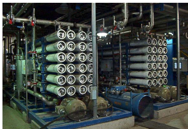
Figure 2: Main level showing the Titan systems
