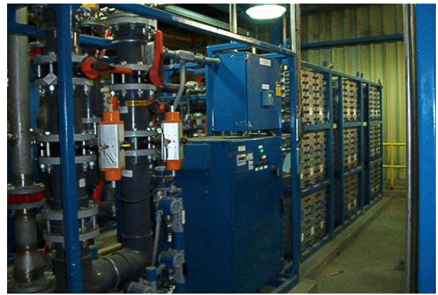
Figure 2: Mezzanine level above the UF and RO membranes, showing E-Cell Stacks
