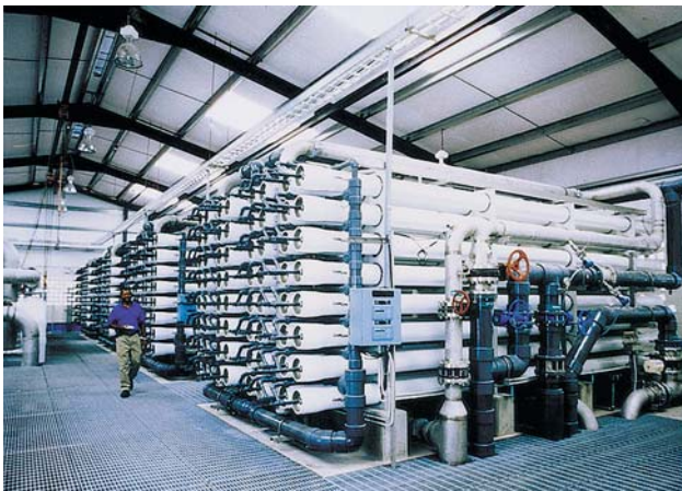
Reverse osmosis technology at the Spring Garden plant.
