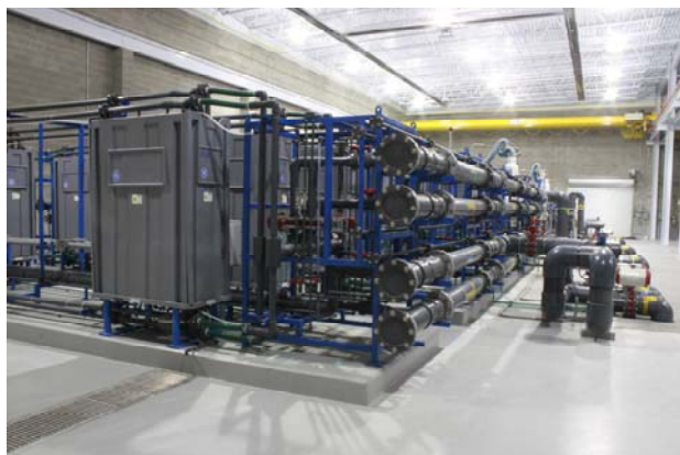
Figure 1: EDR treatment facility at Magna Water District
