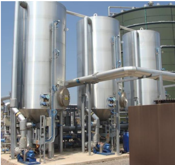
Figure 1: SUEZ’s Re:Heat* heat recirculation system
