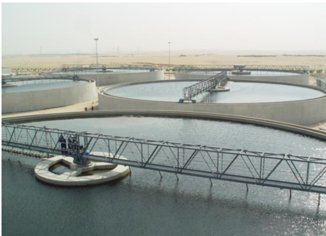
Figure 1: Wastewater treatment facility at Sulaibiya near Kuwait City
